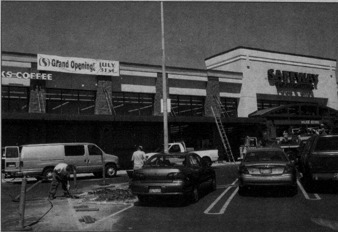
Landscapers put the last finishing touches on the newly constructed Safeway, located at West 18th Avenue and Oak Street. Adam Jones Emerald
