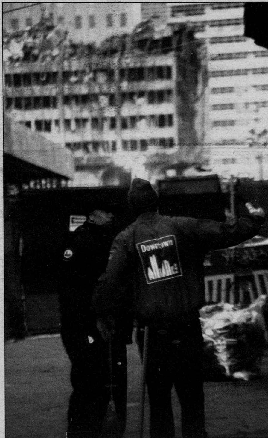
World Trade Center Building No. 7, ruined in the Sept. 11 attacks, is in the demolition process. Some city workers have yet to be given jackets that feature New York's new Twin Tower-less skyline.
