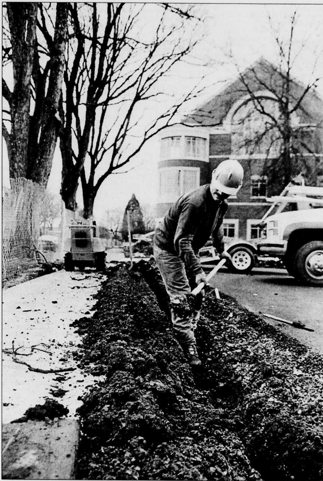
Dave Cheek, an employee of Nature's Landscape, digs a ditch for an irrigation system at the new law center Tuesday afternoon.
