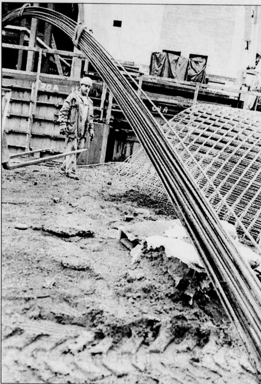
Scott Joy supervises as metal rods are lifted at the Esslinger Hall construction site Tuesday afternoon. Amanda Couvan/Emerald
