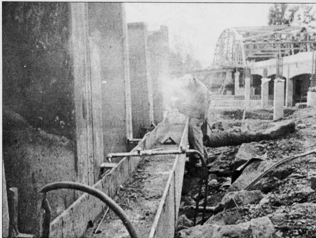
Mowat Construction worker Garry Ray of Stayton welds at the foot of the Ferry Street Bridge Friday afternoon.
