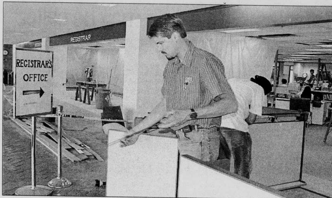
Vince Yarbrough, contract worker for Office World, assembles new cubicles on the second floor of Oregon Hall. The second floor had not been worked on since it was first inhabited in 1973.
