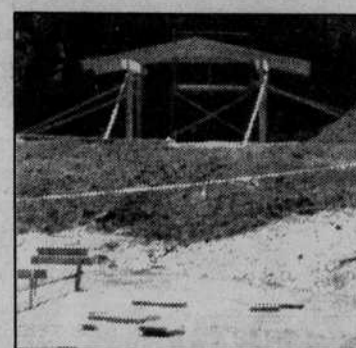
ANDREA DEYOUNG/EMERALD The UO Design/Build class is creating an environmental center, leading to a new outdoor shelter and classroom at a local school.
