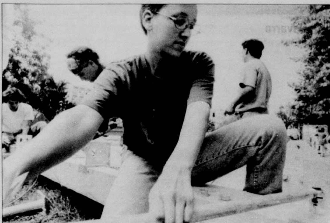
Christina Wikner uses an extension bar to tighten a connector plate bolt to the main beam. BRIAN HENDRICKSON/Emerald
