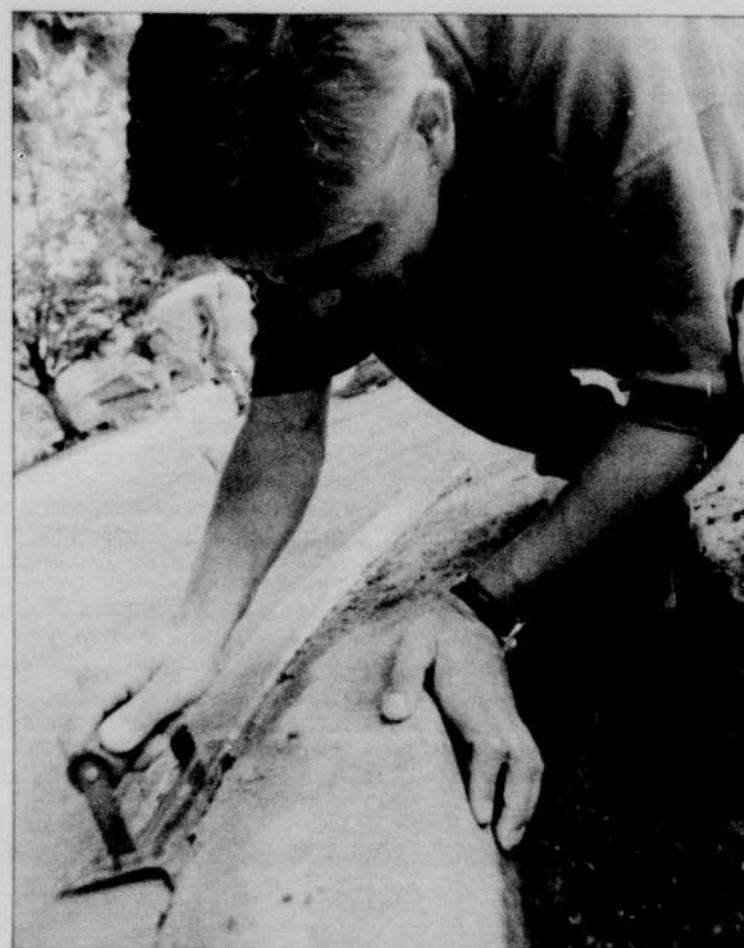
Using a trowel, Jake Freauff smooths the corners on a new sidewalk that will connect the bridge to the existing walkways and crosswalk. BRIAN HENDRICKSON/Emerald
