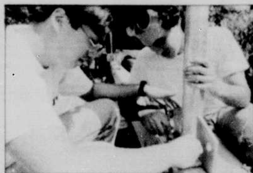
Students Boon Lim and Chris Torlasco align steel connector plates that will link the main bridge beams.
