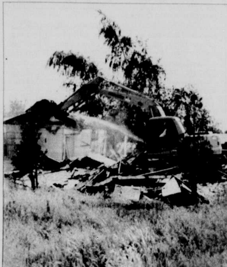
Crews resumed tearing down the Amazon Family Housing complex Wednesday, after a temporary stay against the demolition was lifted.
