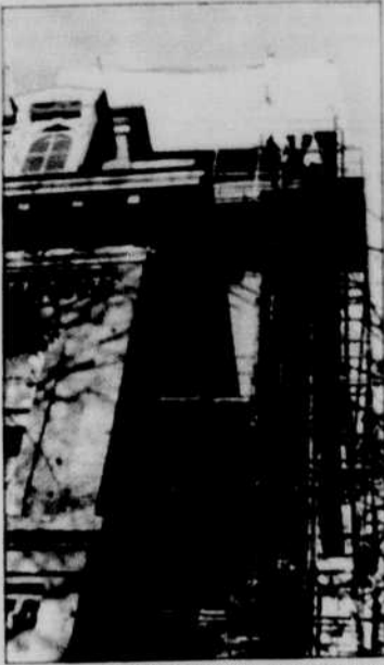
NORMAN MESMAN/for the Emerald The scaffolding and tarps on Deady Hall are part of a preservation project aimed at saving the east tower, which has been threatened by chronic leaks.
