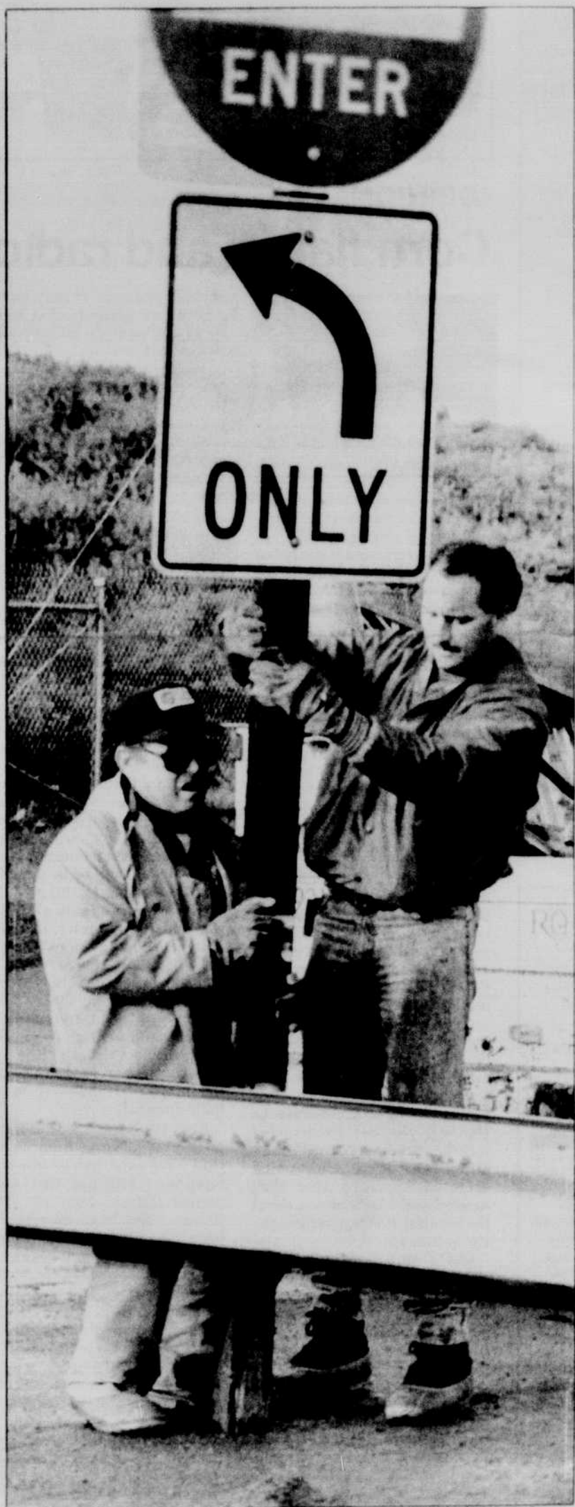
City of Eugene Transportation Division workers Charles Lange and John Ledgerwood erect a new sign and barricade at the corner of Clark and Washington streets.
