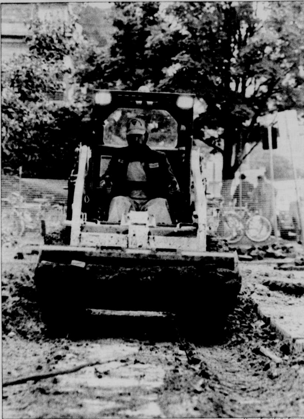
Gerald Henry, with the UO Physical Plant, uses a bobcat to remove the sidewalk in front of Straub Hall. A new sidewalk will replace the old cracked and damaged one.
