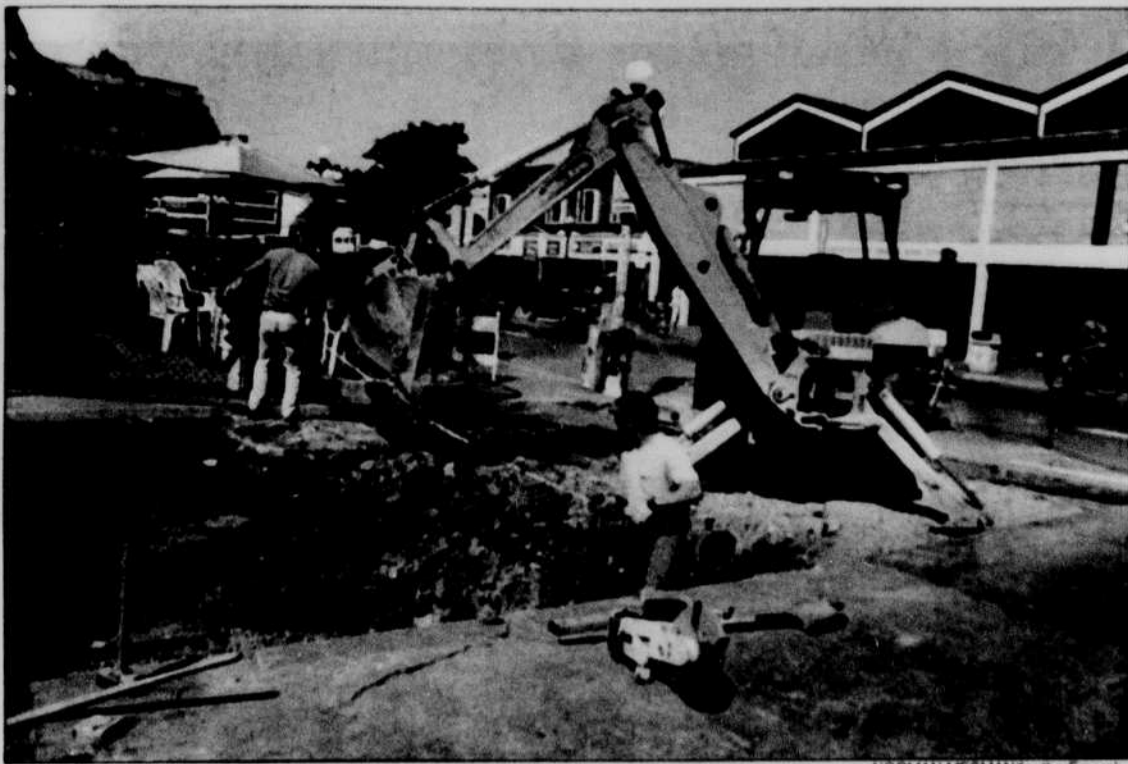
Taylor's College Side Inn is directly affected by the construction on Kincaid Street.
