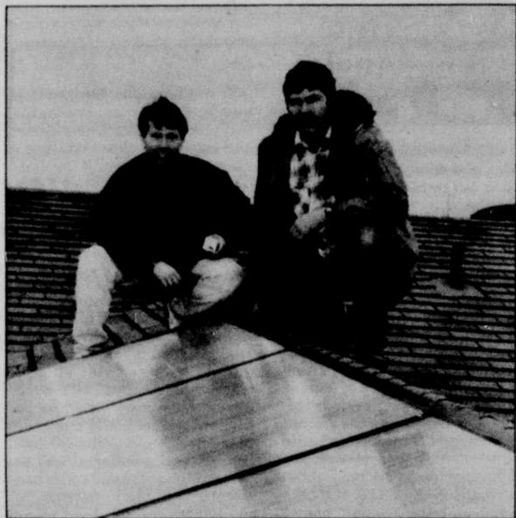
Courtesy photo Paul Israel (left), owner of the American Solar Network, sits atop the roof of client Ken Nanness with a flat EPDM panel.
