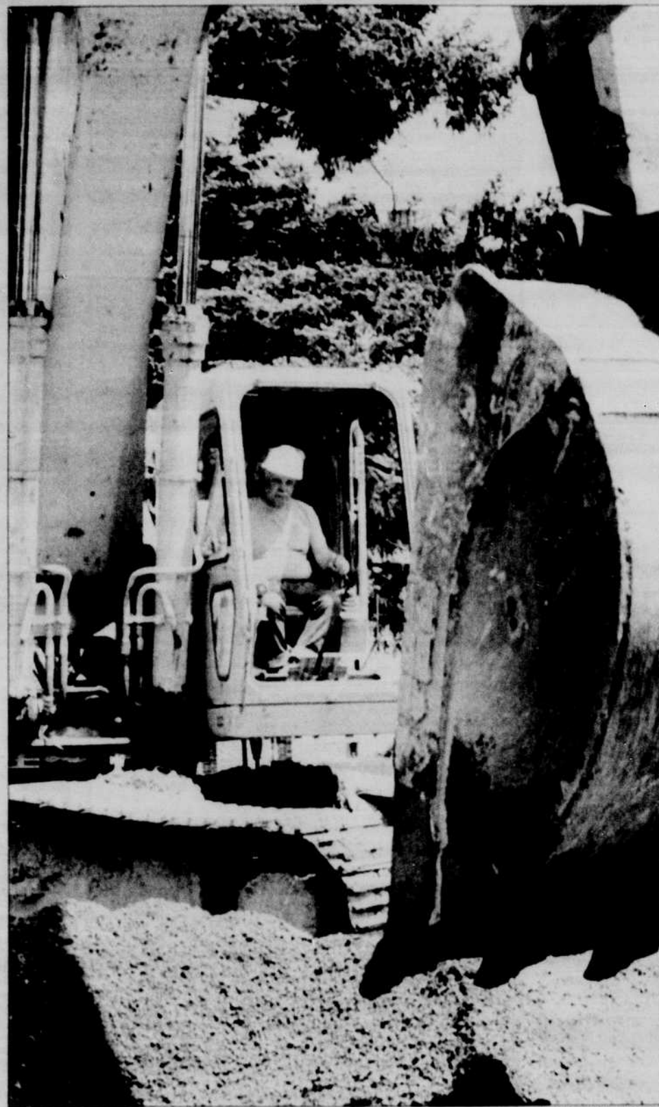
Bill Lyman of Eugene Sand & Gravel shovels gravel into the hole dug for a new sewer line in front of Esslinger Hall.
