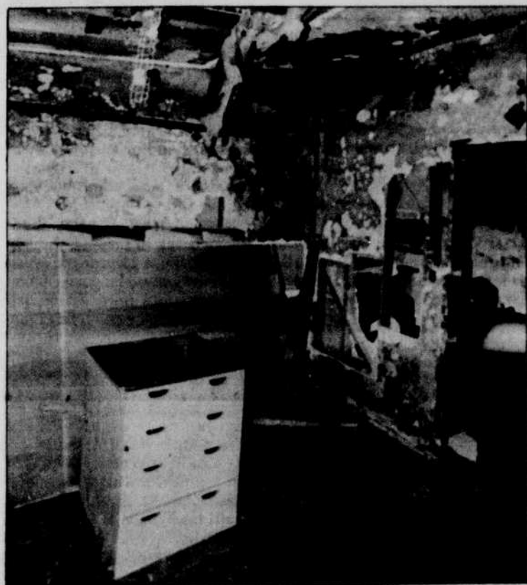
Although the original fire-damage estimate for the Sigma Phi Epsilon house was $35,000, members say costs will be $110,000.
