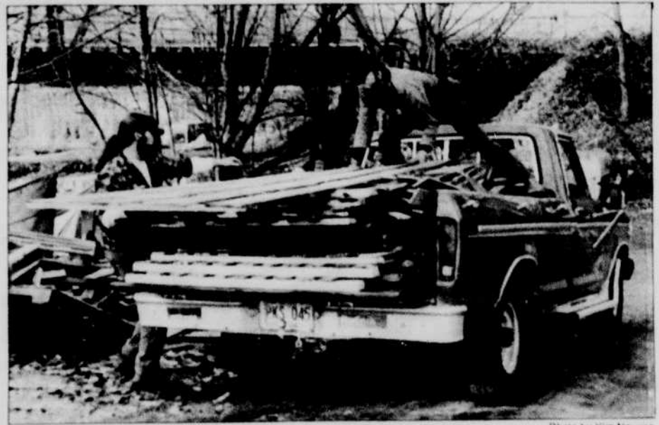
Photo by Kim Nguyen James Nealy (left) and Mac McFadden unload pallets that will be used in building the new Armitage Park tent village for the homeless.
