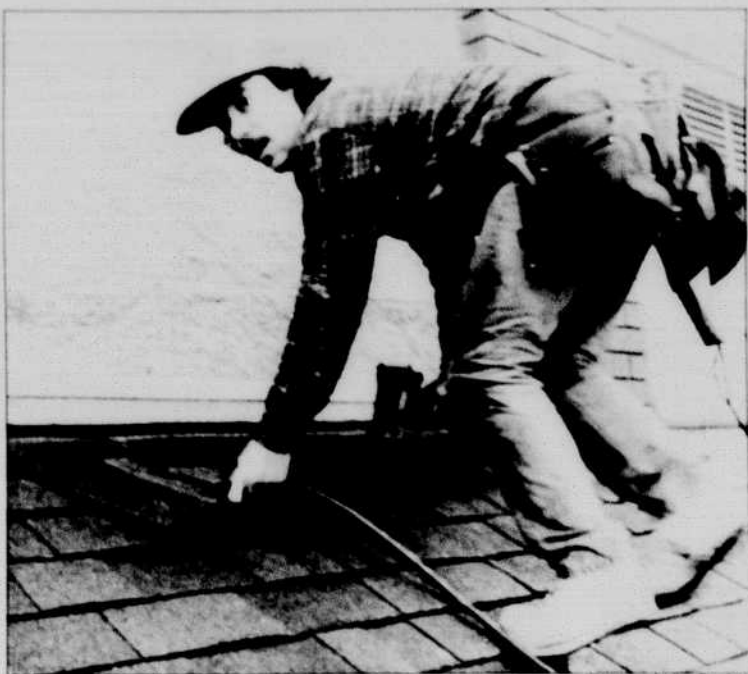
A construction worker adds some finishing touches to the Bowerman Building at Hayward Field. Architect Johnathan Stafford said the building should be completed by spring.
