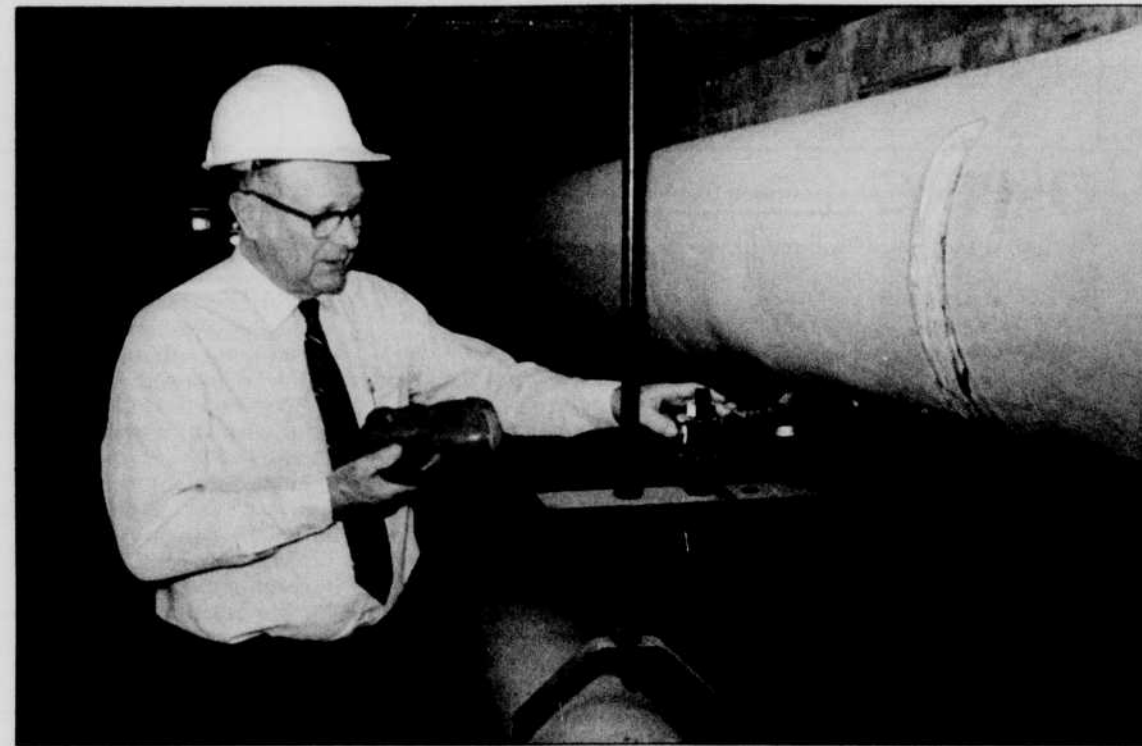
Harold Babcock, University Physical Plant director, inspects a steam valve during a recent tour of the service tunnels that run under the University grounds.
