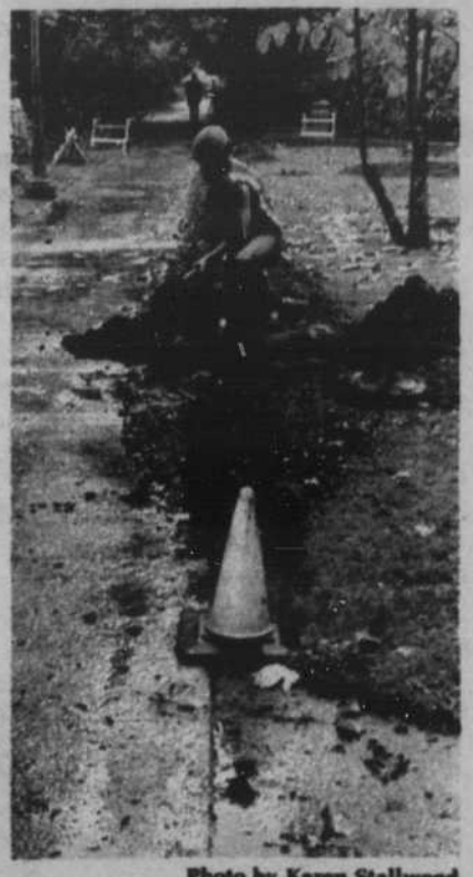
Photo by Karen Stallwood A Physical Plant employee installs sprinkler pipe between Lawrence and Deady Halls.
