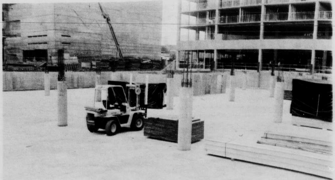
Emerald photo Work on the Hilton Hotel and the Performing Arts Center in downtown Eugene should be completed by November 1982, according to city officials.
