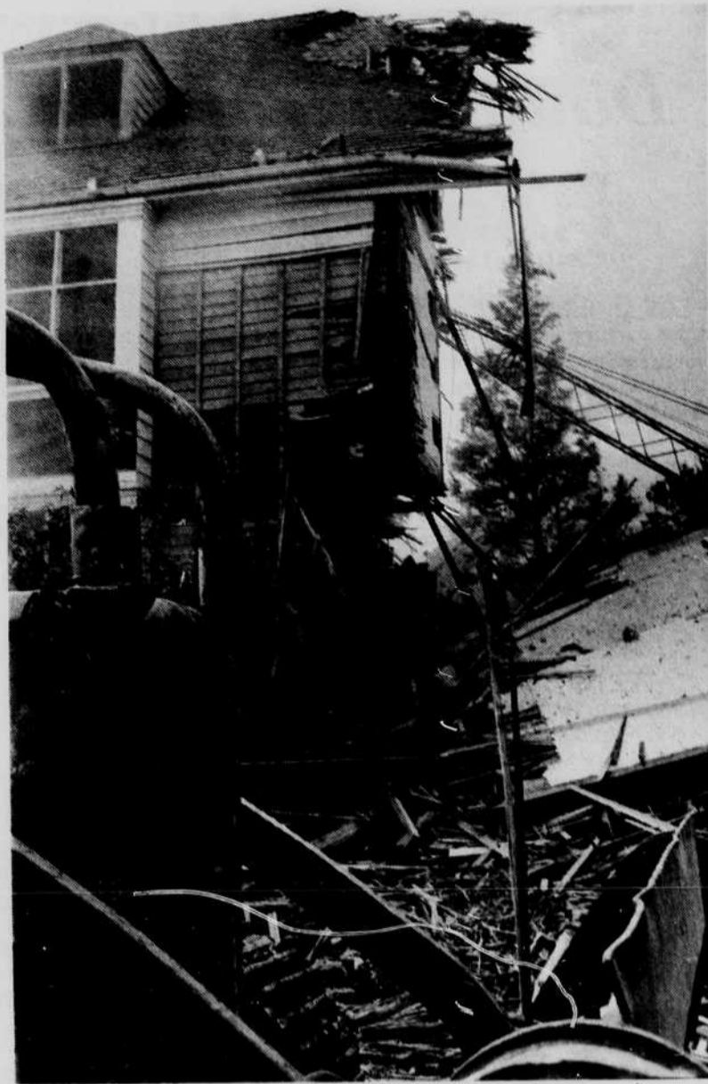
Fall rush at this former sorority and boarding house meant that workers were in a hurry to demolish the structure, which they did last week. Building was located at 13th and Alder St. Photo by Peter Weinrobe
