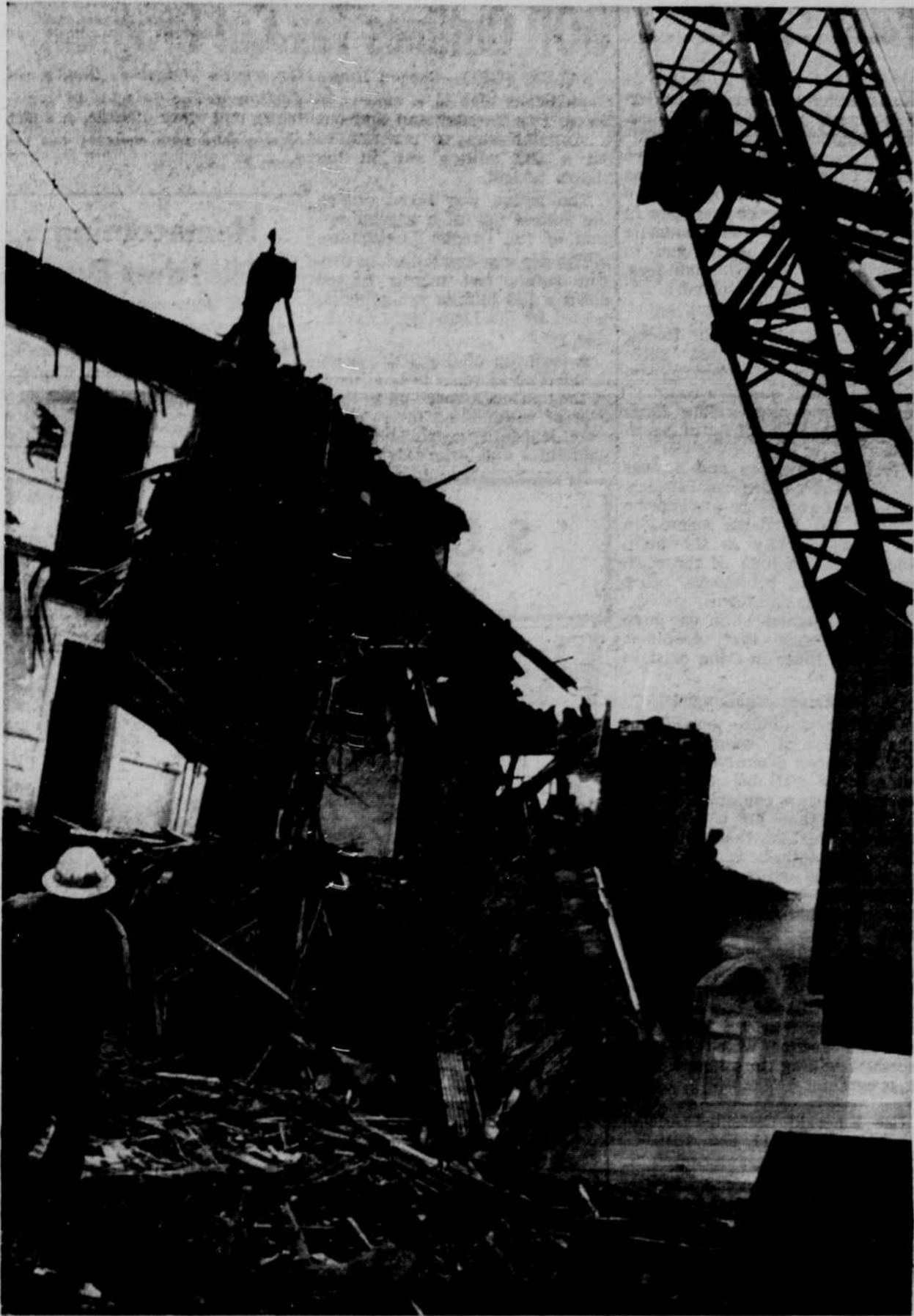
WORKMEN were occupied in demolishing and cleanup work at the former Sigma Chi house this week. While the fraternity is building a new house, members are housed in temporary quarters. Photo: Bigham.
