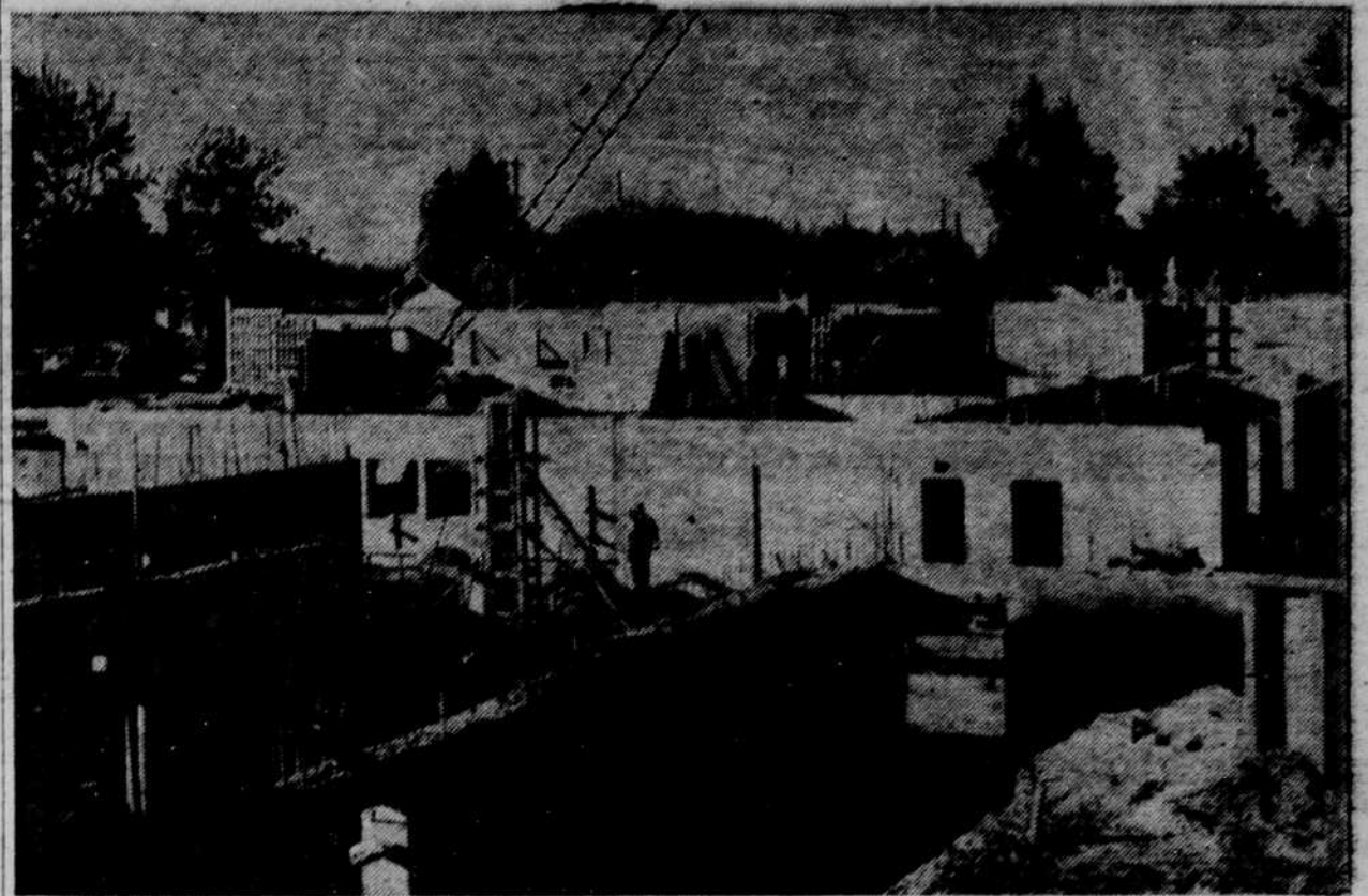
CAMPUS HOUSING SITUATION is getting lots of attention. Mostly freshmen occupy all dormitory space available this year, and a record number of students are living off-campus. This 13th and Agate construction site is the first of ten dormitories to be built in the next 10 years if the bond measure meets approval in November's elections. (Emerald staff photo by Dave Sands.)
