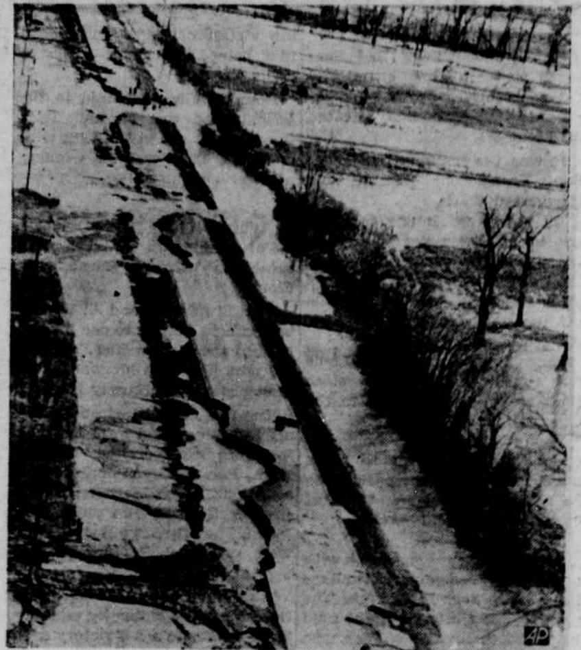
FLOOD-NIBBLED HIGHWAY — Hungry flood waters nibbled huge chunks out of this stretch of pavement on a highway south of North Bend, Nebraska. This low aerial shows how the highway looked after the high water subsided.
