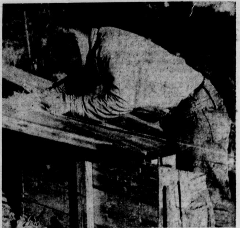
AS SOON AS the steel letter was in place, the welding of the four sections was begun. Ken Opager from Eugene Truck and Machinery Co. donated his time to do the welding.
