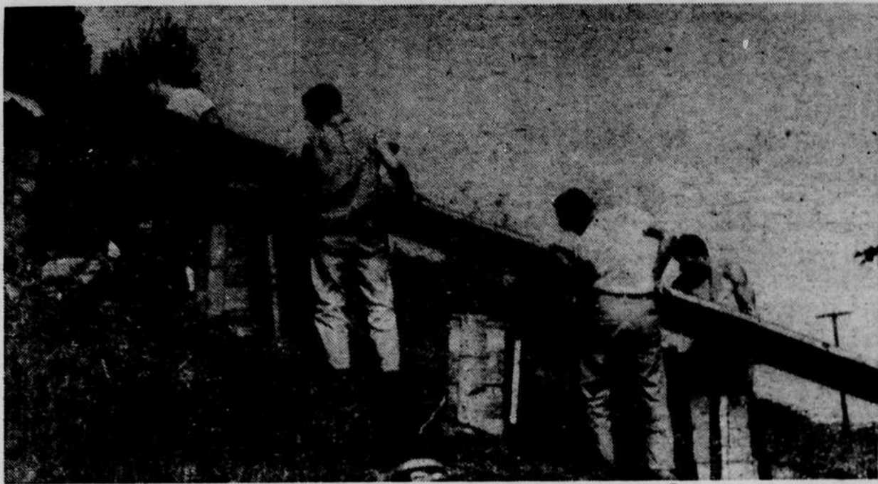
THERE WASN'T MUCH to see on the "O" construction until the one and one-half ton steel letter was set in place. The sections weighing from 750 to 850 lbs. were set in position by members of Alpha Phi Omega on Friday before Junior Week.
