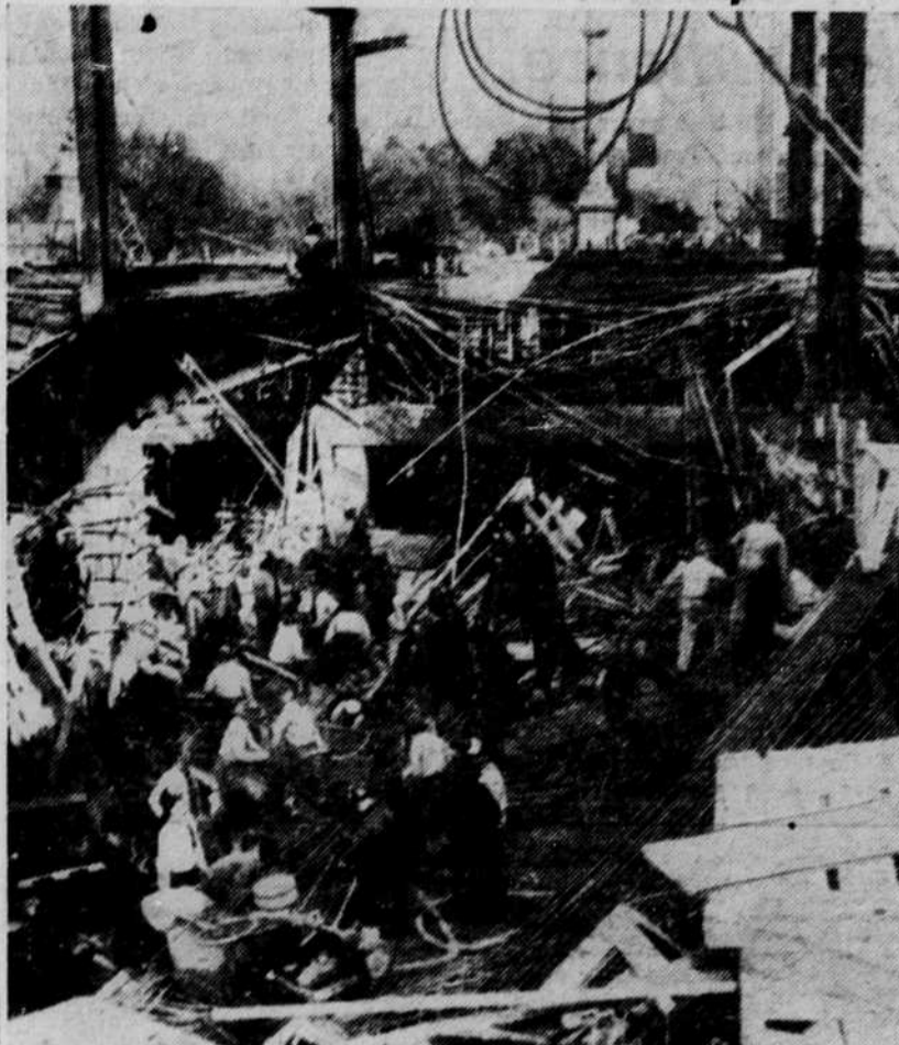
POLICE, FIREMEN and construction workers hunt through wreckage that crashed 22 feet when center section of exhibit floor of New York's new coliseum collapsed during construction work, May 9. View looking east shows the Christopher Columbus statue, upper center, in Manhattan's busy Columbus Circle. Of 1000 at work on the building when the collapse occurred, one is dead and at least 50 are missing. (AP Wirephoto)
