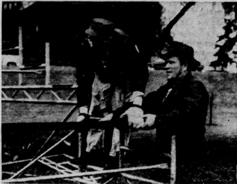
WITH WORK ADVANCING well on the bleachers for the Canoe Fete, Jerry Maxwell, bleacher set-up chairman, and an unidentified member of the physical plant lend a helping hand with the construction.
