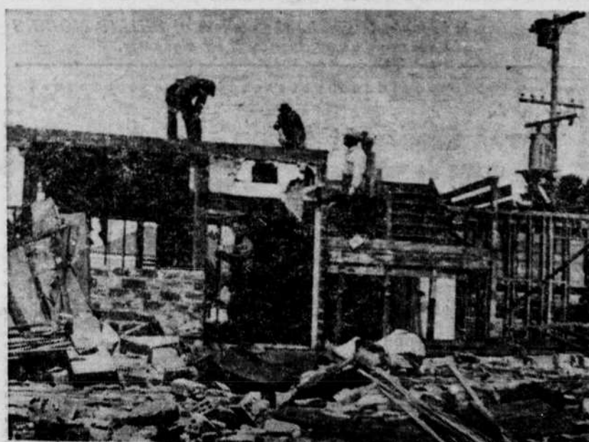
COMING DOWN is Vets' Dorm number 1, abandoned this fall after being termed a "fire hazard" last spring by Eugene Fire Chief Ed Surfus.
