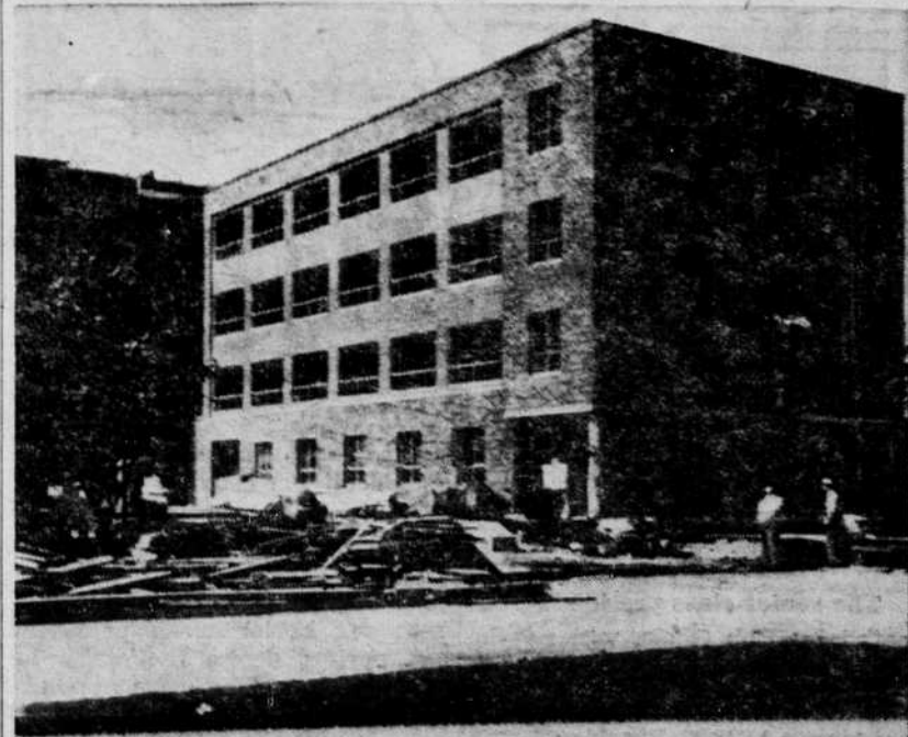
GOING UP on schedule is the $1,250,000 men's dormitory, Virgil D. Earl hall. University officials expect the modern addition to John Straub hall to be ready for occupancy by September, 1955.
