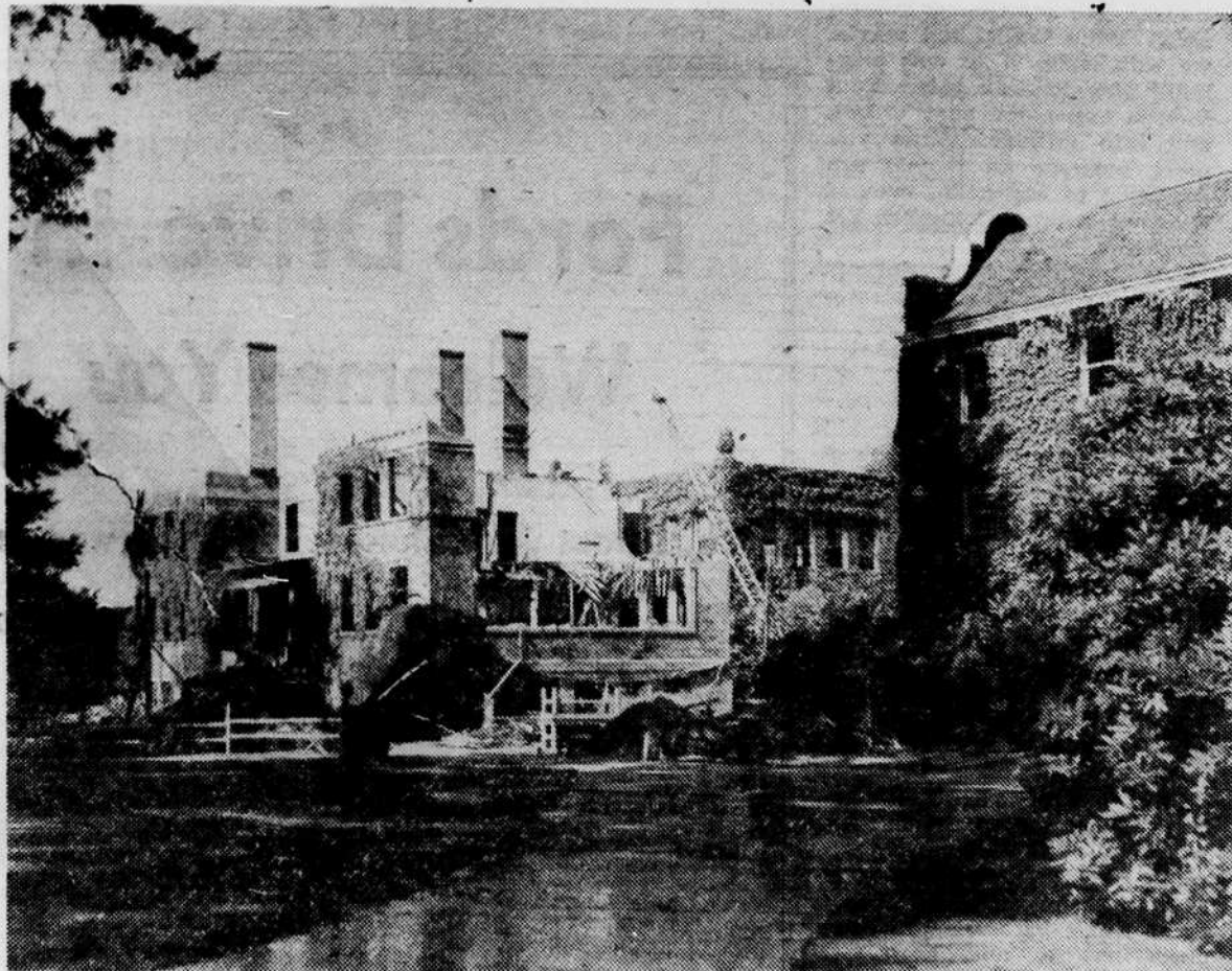
McCLURE HALL as it appeared in early August when it was being razed to make room for the new $559,000 journalism building which will be completed in late 1954. The first permanent building ever to be torn down on the campus, McClure was completed in 1900 at a cost of $28,000. It was the third oldest building on campus.
