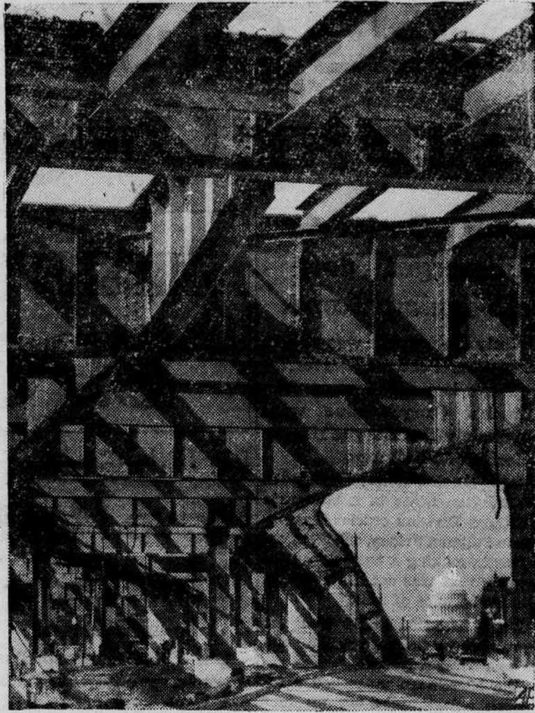
THE CAPITOL at Washington stands framed by the steelwork for the new South Capitol street bridge which will span the Anacostia river in November. (AP Wirephoto)
