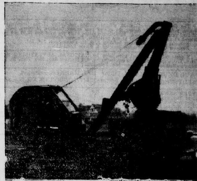
This picture of the excavation of the Humanities building basement . . . was taken several weeks ago. Now work on the cement foundation pouring is progressing rapidly.
