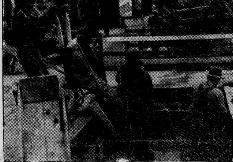
Emerald Photographer Bill Scott ... caught the above pictures of construction work on three campus projects for which $253,170 is being spent. The Humanities building (being excavated, upper left) will cost $165,455. Hayward stands (upper right), $40,715. Heating and service tunnels (below), about $47,000. Engraving by Lloyd Tupling.
