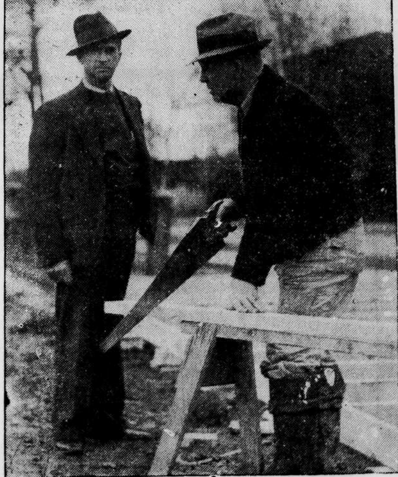
Al Stien and Ed Hulse . . . contractor and carpenter, on the job last week to begin preliminary work for the building of Oregon's new $160,000 Humanities structure. University students on their way to register today will see excavation work begun. The building will be located across the street from Commerce and will be completed by next fall.
