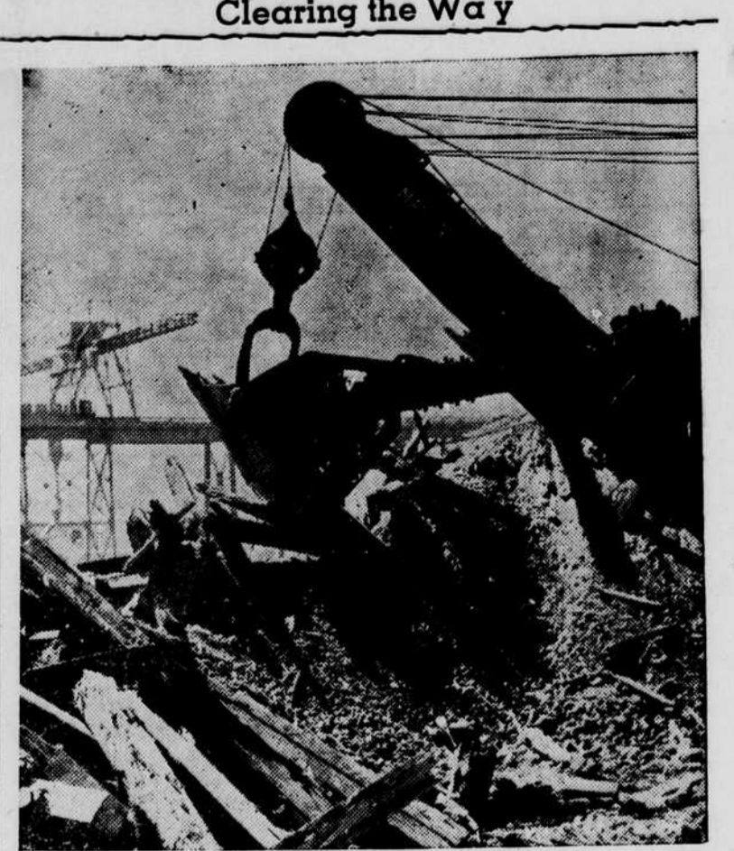
Scoping the cofferdams at Grand Coulee is the big shovel above. Largest cement dam in the world, this biggest of government projects was inspected recently by Franklin D. Roosevelt on his western tour.
