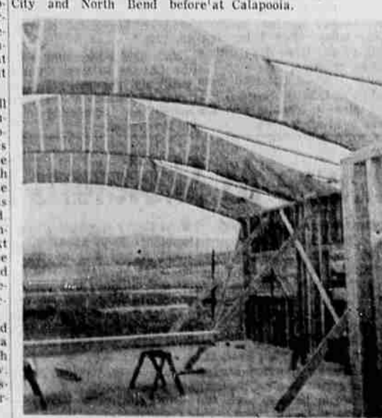
LAMINATED BEAMS, as shown above, will support the roof of the new Calapooia Free Methodist Church now under construction west of Sutherlin. The church is being constructed on a site between the Umpqua road and Highway 225.
