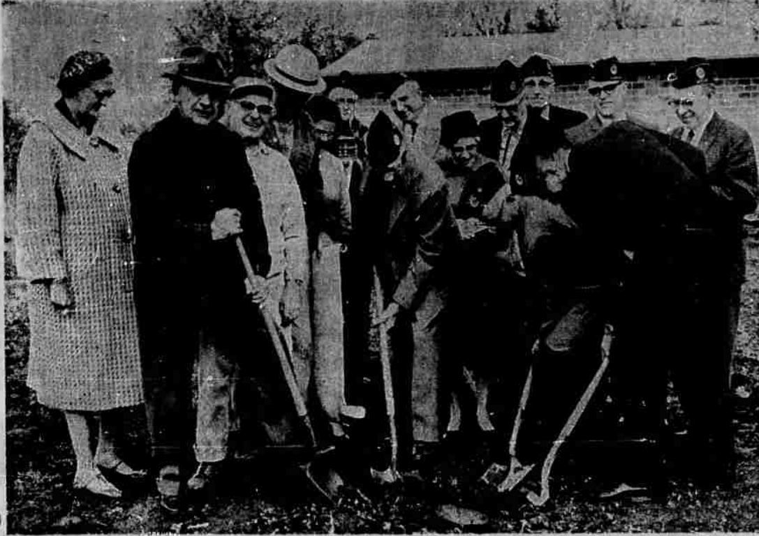
BIG OCCASION — Four officers of the Umpqua Post of the American Legion turned over the first shovels of dirt to start construction of a new Legion home at 406 SE Oak Ave., Roseburg. Those with shovels, from left, are: Noble Goettel, finance com-
