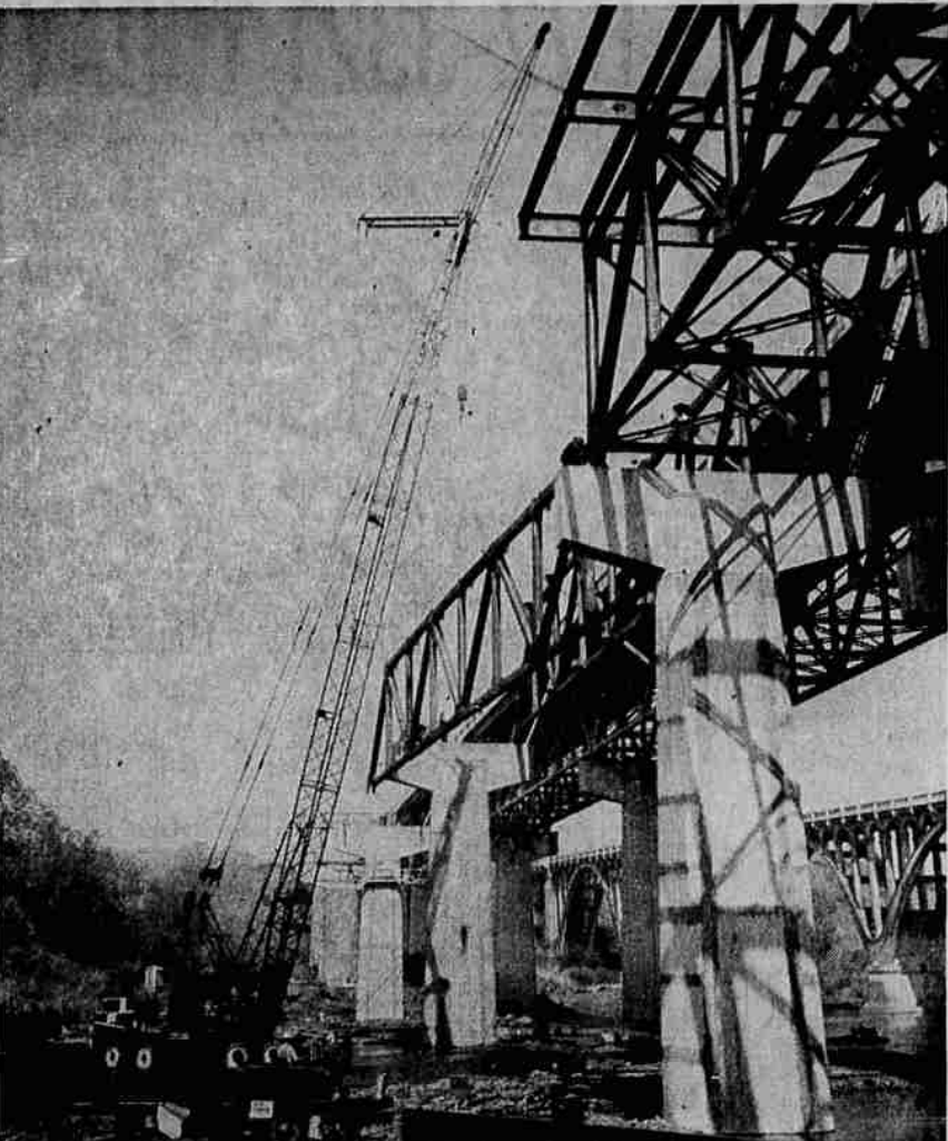
WINCHESTER BRIDGE —A 75-foot high crane, capable of lifting 75 tons, hoists into place steel girders for the new Highway 99 bridge at Winchester crossing the North Umpqua River. This bridge is a duplicate of the existing bridge, and will carry south bound traffic in the four-lane highway construction project now under way. Main piers crossing the river are in place, and steel trusses being erected. This portion was completed early in order to eliminate difficulties with high water later. Four more piers to the south remain to be constructed. June of next year is the completion time table, and work will continue during the winter months. Workman Construction Co. of Canby, has the contract. (Chris' Studio)
