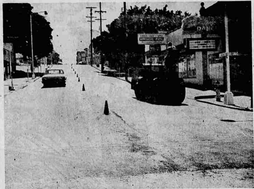
BUSINESS AREA STREETS began getting new surfaces this week in connection with a street "redecking" improvement project. Work on the streets will continue until about the middle of next week. Above, work progresses on SE Jackson St. between Center and Douglas avenues. Eight other streets are involved in the project. Added to the original list were Vista Ave. between Overlook and Chadwick. When work begins on particular streets, "no parking" signs are installed. Cars may be hauled away if they are left by the owners on the posted streets. (News-Review photo)
