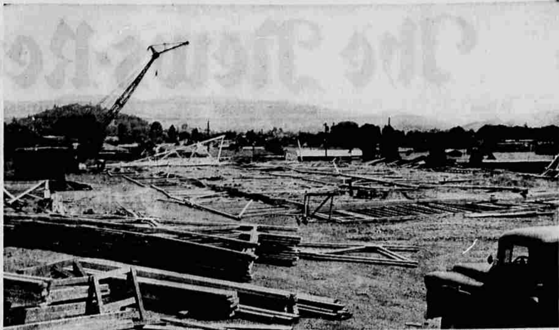
GOING UP AGAIN — Carpenters at the site of the new Roseburg Seventh-day Adventist School began the job Friday of raising the framework of the school on which construction started about a month ago. Earlier Friday, supporting trusses on the framework gave way and the entire structure sagged to the ground. A crane here is shown lifting the trusses out of the tangle. Very little damage resulted from the mishap. (News-Review photo by Chris)
