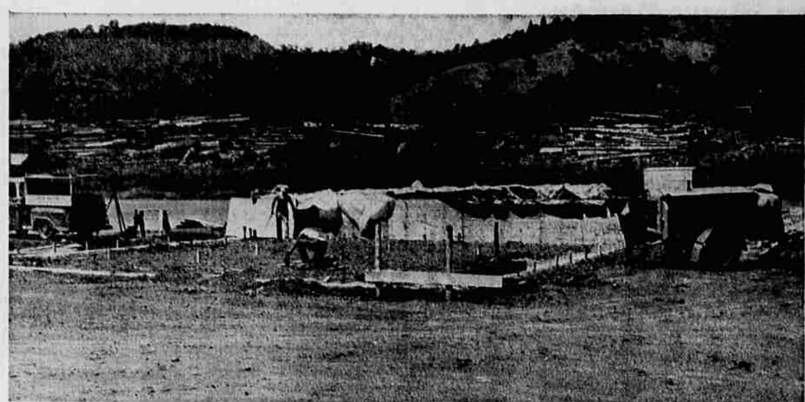
FOUNDATION is being prepared for a new building on NE Diamond Lake Blvd. just east of the Roseburg Bowl, which will be the headquarters for the first liquid oxygen filling station installed west of the Mississippi River by the Air Reduction Pacific Co. (Airco). The plant, under Airco franchise, will be operated by Oregon Welding Supply Co., and will employ about 18 persons, servicing South-
