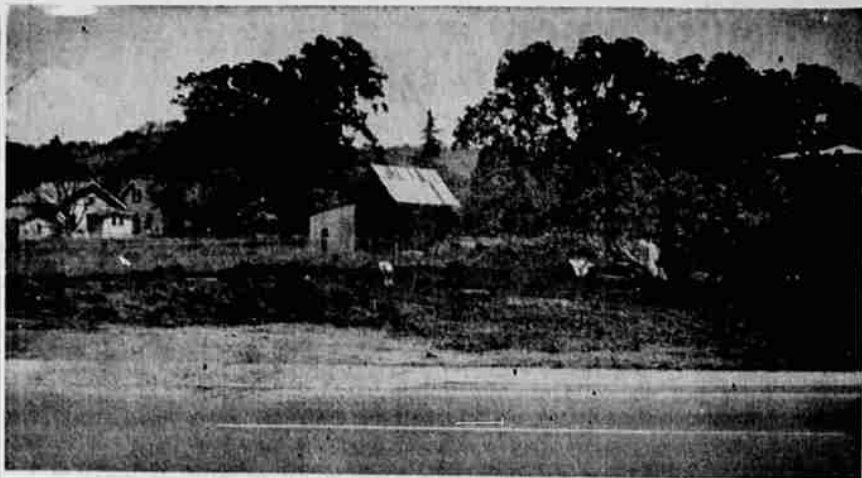
EXCAVATION AND GROUND LEVELING was started this week to make way for construction of a new ice cream center, which Arctic Circle, Inc., plans here. The firm, out of Salt Lake City, which has many franchise outlets in the west, has taken out a building permit for $15,900. The location is on W. Harvard Ave., just west of the Washington Ave. Bridge. (Chris' Studio)
