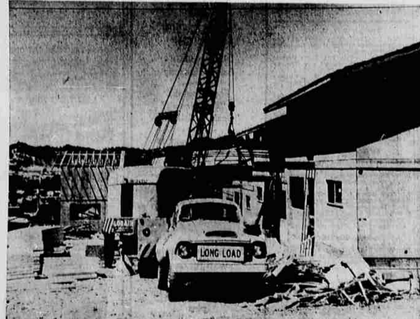
CONSTRUCTION on the nine-unit apartment building by Ray Hill and Neal Flanagan of Roseburg on W. Crestview Ave., is moving along rapidly, as the photo above indicates. The Engle and Person crane was called in to move material to one of the levels of the multi-level building. The apartment house, which will have numbers ranging from 2332 to 2348 Crestview, is estimated to cost $61,700. Building permit on the work was taken out May 2 from the Roseburg Building Department. The outside walls are prefabricated, but the owners are putting in their own inside work. The apartments are located behind Mark's Shopping Center in the West Slopes Addition area. (News-Review Photo).
