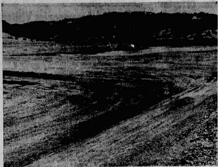
WORK IS NEARING COMPLETION on the settlement ponds for the Green Sanitary District and should be wrapped up by next week, according to the contractor, Selmar Hutchins. Pressure and arterial lines will be in by September or October. The contract calls for three ponds and all lines at a cost of over $402,000. Some 63 men are employed on the job, most of whom are local.
