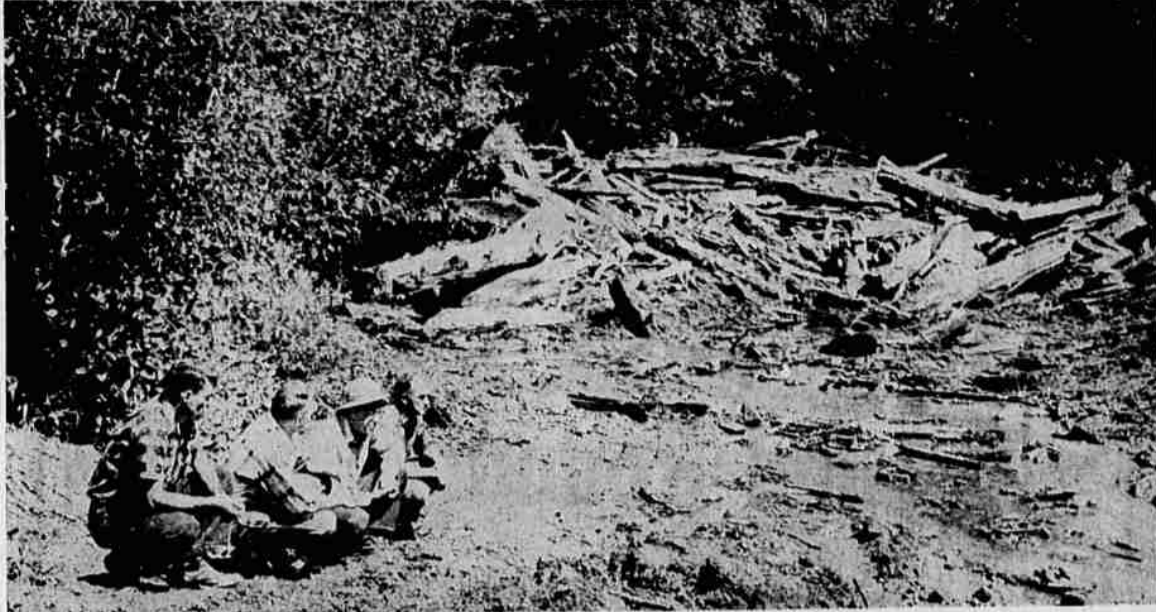
NEARING THE END — The Umpqua - Smith River watershed stream clearance project of the Oregon State Game Commission, jointly sponsored by affected land-owners, is nearing completion. The project involves about 18 miles of log jams. Shown is the removal of the Weatherly Creek drifts. (Down Peseau photos).
