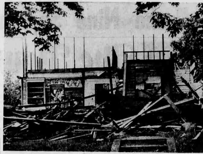
SCENE OF DESTRUCTION is one of many along the route of the west approach to New Washington Ave. Bridge. Several houses are being torn down and others are being moved to make way for the approach. Roseburg Paving Co. has the route construction job, which it bid at $88,402.
