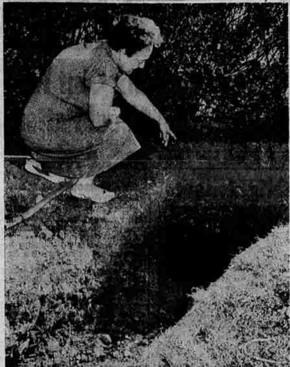
DO-IT-YOURSELF DITCH at 2958 Harvard Ave., is the work of Melvin B. Rodgers, a Forest Service employe who dug the ditch and tunneled under a hedge to connect his home with a new sewer line installed along Harvard Ave. Mrs. Rodgers is shown examining her husband's work, which is now complete except for installation of the pipe. (Paul Jenkins)
