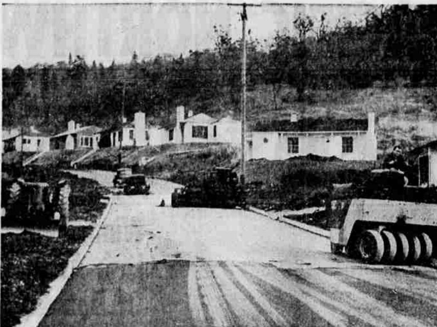
PAVING OF SEVERAL STREETS got under way in the Cloverdale section Thursday. About five days of paving are scheduled, weather permitting. Roseburg Paving Co. is doing the work on NE Brooklin Ave. from just west of NE Morris St. to NE Todd St. and north on Todd to Alameda. Morris, Hollis and Todd are also being paved to their ends south of Brooklyn. Curbs and gutters are being put in on other streets, and paving of the remainder of the area will resume in the spring. (See story Page 6.) (Paul Jenkins)
