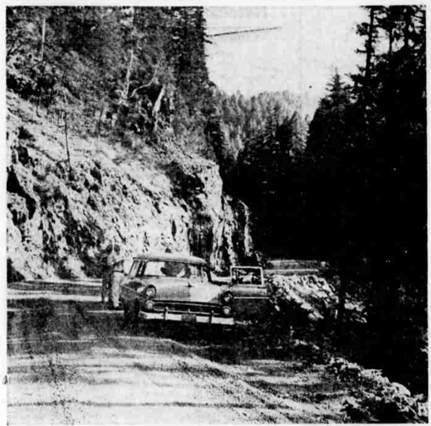
BETTER ROAD , constructed by Copeland Creek and across Fish Creek in the Umpqua National Forest is providing quicker access to timber sales on the Diamond Lake District of the forest. The road was straightened and widened by Roseburg Lumber Co., a timber purchaser. The company also is building a road into the Rhododendron Ridge country that eventually will provide a link between the North Umpqua and South Umpqua watersheds. Another road is being extended up Copeland Creek and eventually will lead to a point near Twin Lakes, which the Forest Service expects is destined to become a major recreation area. (Paul Jenkins)
