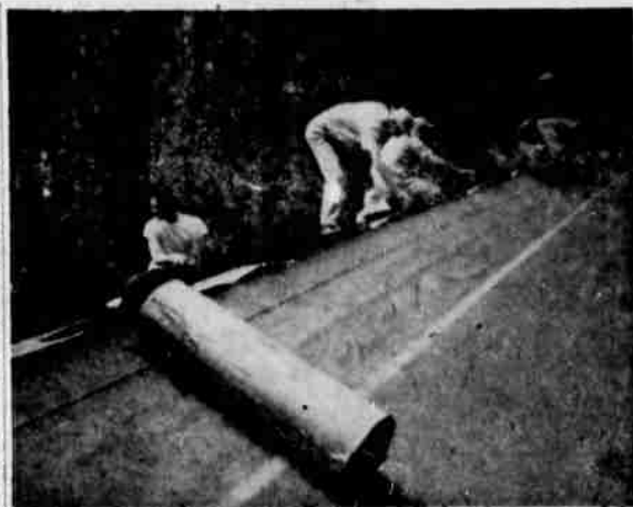
CAMP TYE was made ready over the weekend by the Roseburg Kiwanis Club and Roseburg High School Key Club for this summer's influx of Camp Fire Girls. Busy members of the club are roofing one of the camp buildings above.
